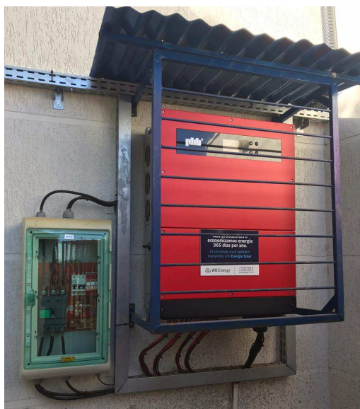
Figura 29 - Inversor PHB35K-MT e QDCA 72.
